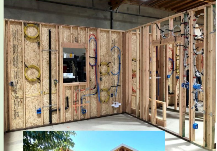
Walls, roof, electrical & plumbing kit
